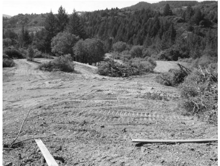
In 2005, the winery site was apparently cleared of trees and chaparral, then graded, without permits.
